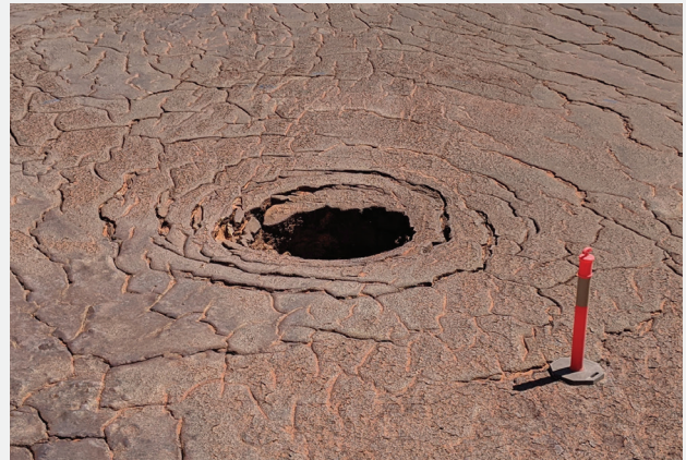
IMAGE: A SINKHOLE FORMING WITHIN A TAILINGS BEACH AFTER SLURRY DEPOSITION. INVESTIGATIONS OUTLINED ITS EXTENT FOR REMEDIATION PLANNING.
